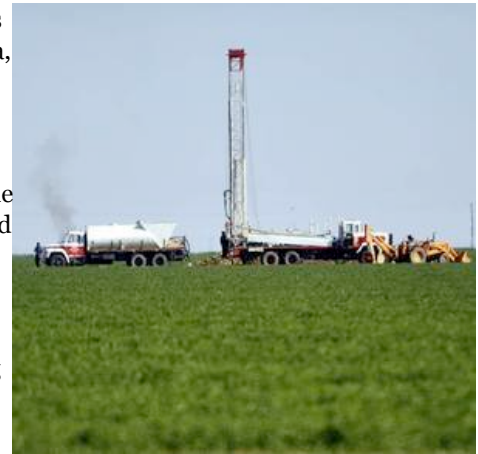
A crew digs a well in an alfalfa field in Dos Palos, Calif., Thursday Nov. 19, 2009. The government is spending $40 million in federal stimulus funds to pull water from underground aquifers in drought-stricken California, even as evidence is growing that the well-drilling boom could degrade the quality of water delivered to millions of residents. - (Russel A. Daniels / The Associated Press) -
